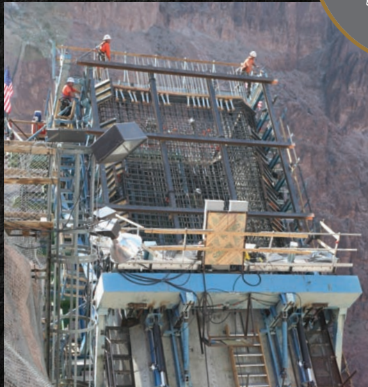
One pier of the Hoover Dam Bypass Bridge nears completion. PHOTO COURTESY SOUTHERN NEVADA LECET.
