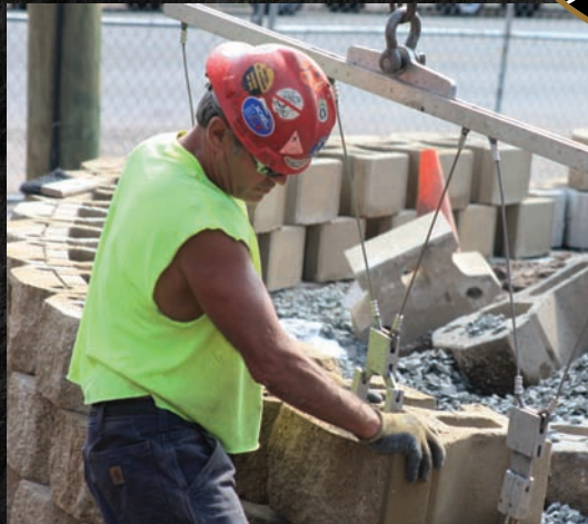
A member of Laborers' Local Union 472 sets block for a retaining wall at St. Joseph's Medical Center in Paterson, New Jersey. PHOTO COURTESY NEW JERSEY LECET.
